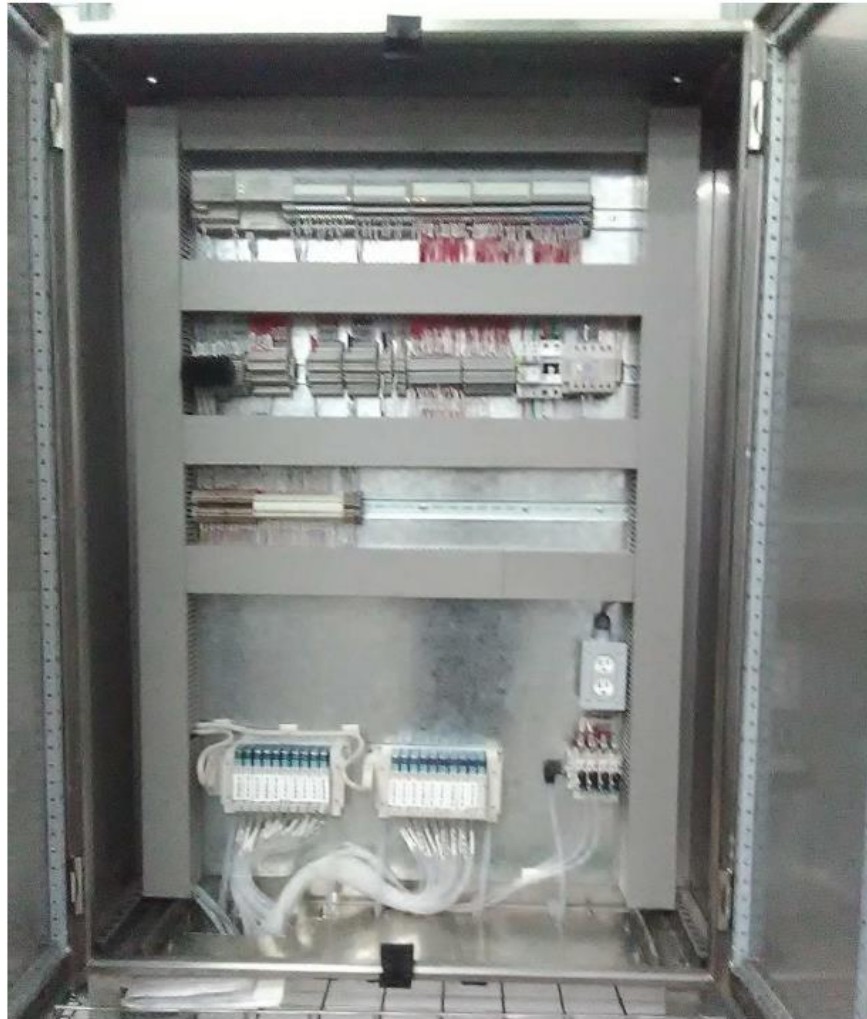
Fig. 4.7 Tablero de control
