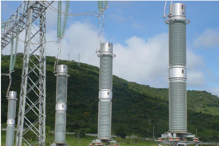
TP's de 400 KV
