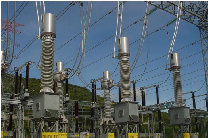
TP's de 115 KV
