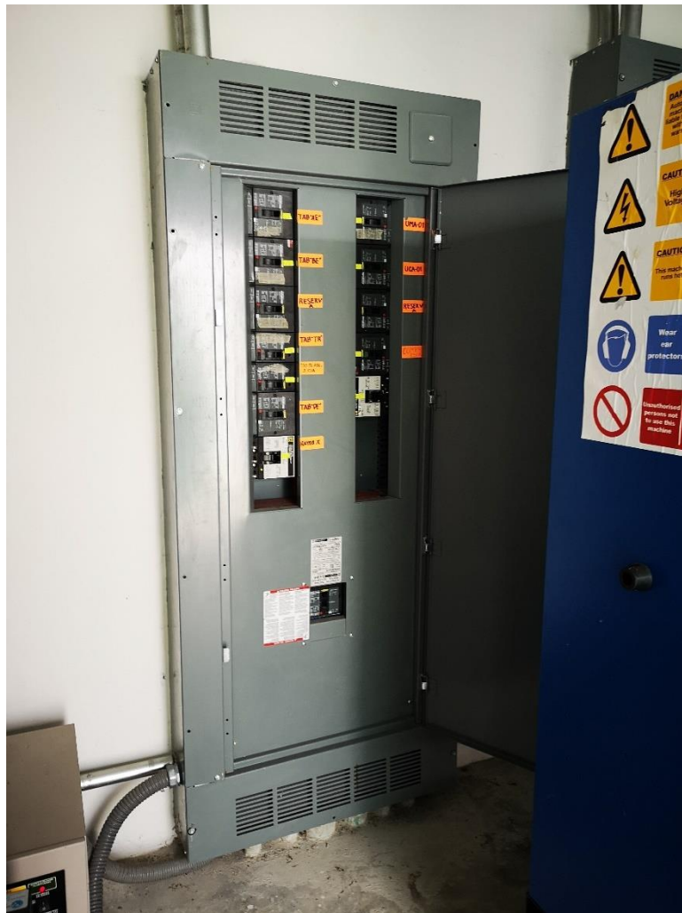
Figura 7. Tablero general normal I-LINE
