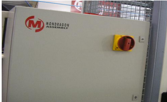
Figura 4.14. Interruptor General del gabinete de control
